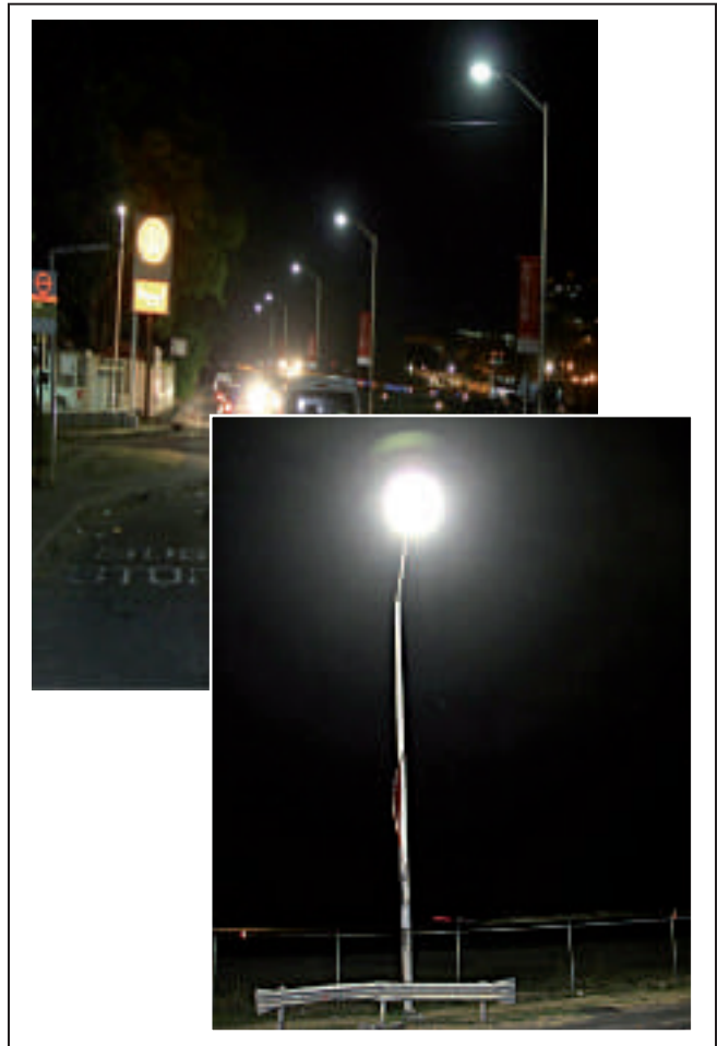
New LED street lights along the John Compton Highway
